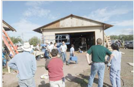
Volunteers work on the nearly finished Franklin family barn. Owner Thad Franklin died last month while working on the project and volunteers on Sunday finished the job. U-B photo by Joe Tierney
